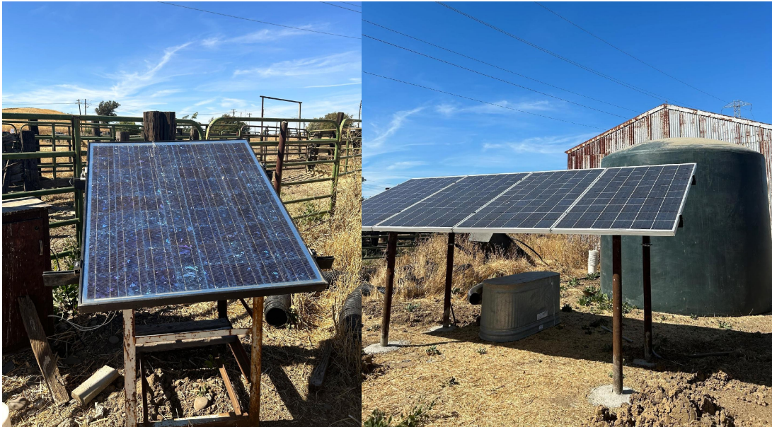
Above (Left): Solar Panel Reuse Project for Electric Fence. Above (Right): Water Pump. 9/2025 – Solano County.
