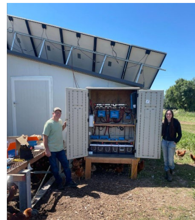
A chicken coop received repurposed solar panels to electrify the building.
